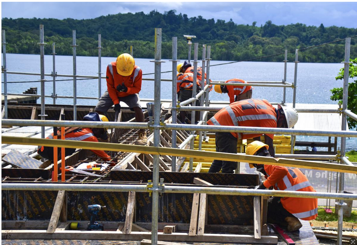
Photo 3 – The new market is rising, with blockwork and roof framing on the new amenities building progressing quickly.
