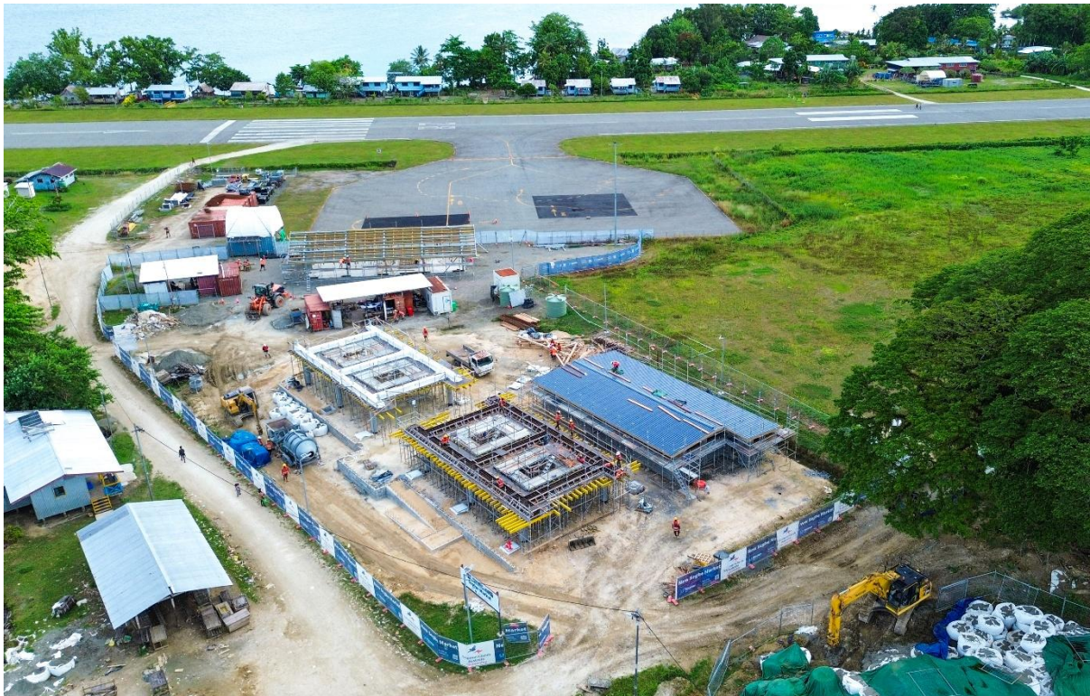
Photo 1 - Over 60% complete! The new market, together with the new Seghe Airfield and terminal projects, are quickly changing the shape and economic future of Seghe.
